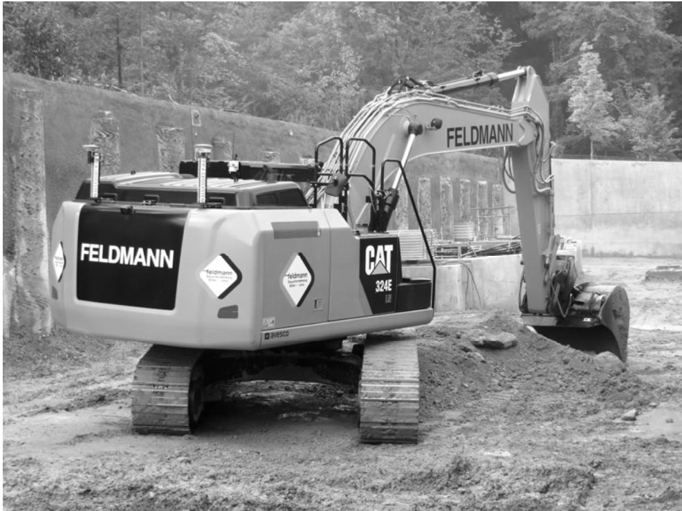
Fig. 3: 3D GNSS machine control system installed on a digger is used at a Landscape Architecture construction site (Zoo Zurich, the new elephant area, October, 2013).
